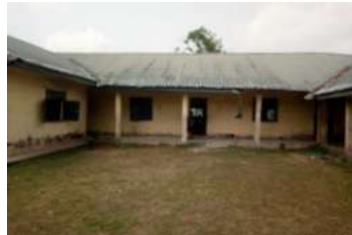
Picture showing the roof condition (CBSS Emeyal (Ogbia))
