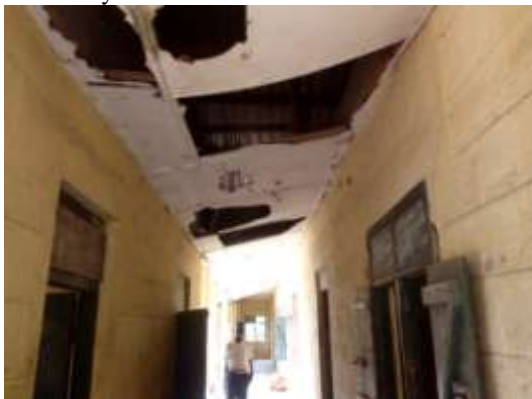
Picture showing the ceiling condition (CBSS Emeyal (Ogbia)
