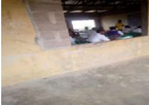
Picture showing the conditions of windows (CSS IGBOGENE)
