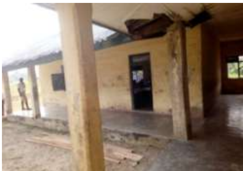
Plate 4.1: Picture showing the condition of floor in the school building (CSS IGBOGENE)
